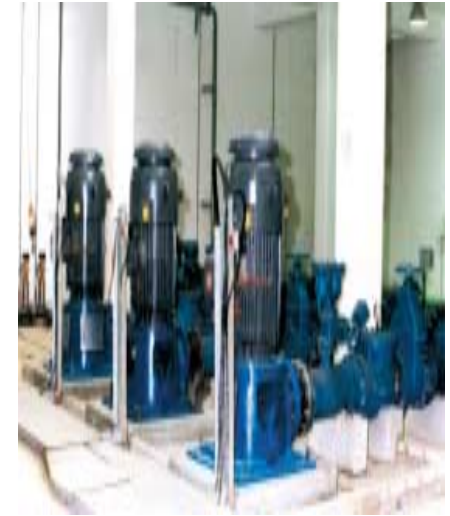
Treated Water Peerless Pumps @ R 22 Sites (MPW)
