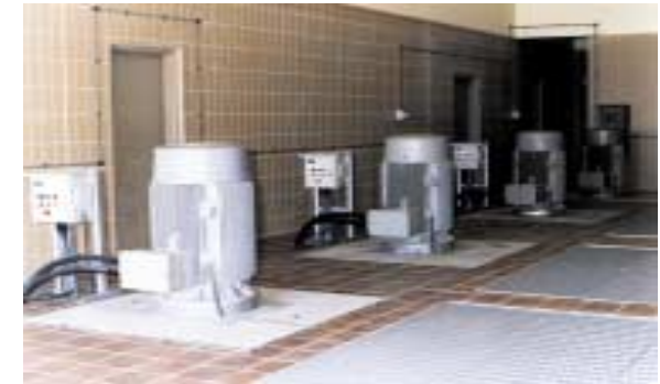
ABS pumps @ Um-Al Hayman Sewage Pumping Station.
